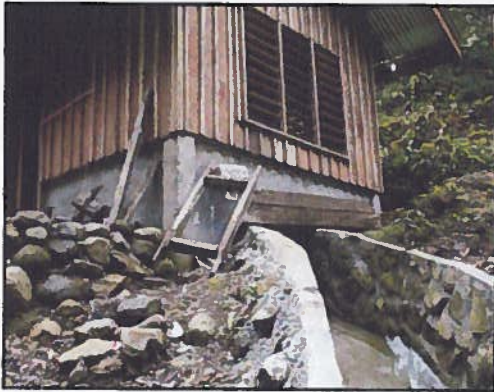
Newly constructed micro-hydro power house, Barangay Old Bulatukan, Municipality of Malasila, North Cotabato, Mindanao Island, Philippines (August 2009).
